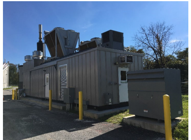
1.25 MW Packaged CHP System SOURCE: PA ENERGY DEVELOPMENT AUTHORITY
